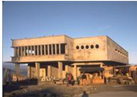
Minor Damage, foundation
