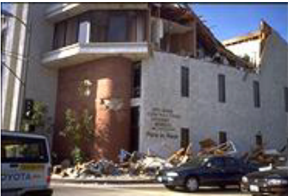
Partial floor collapse
