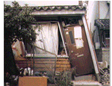
Framed House Shear Failure
